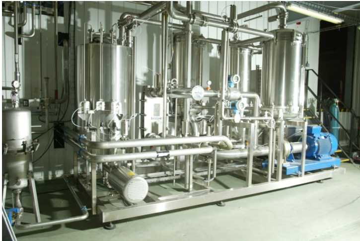
Ceramic Crossflow Filtration Plant
