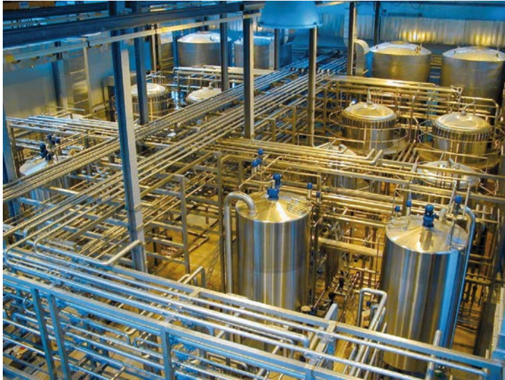
Candle filter plant for filtration and stabilization of Beer
