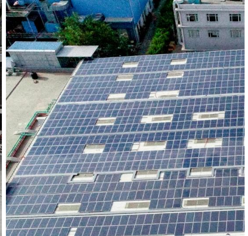
Sustainable power sources Total photovoltaic capacity at kWp 1'224 Solar cells at Bucher Hydraulics, India
