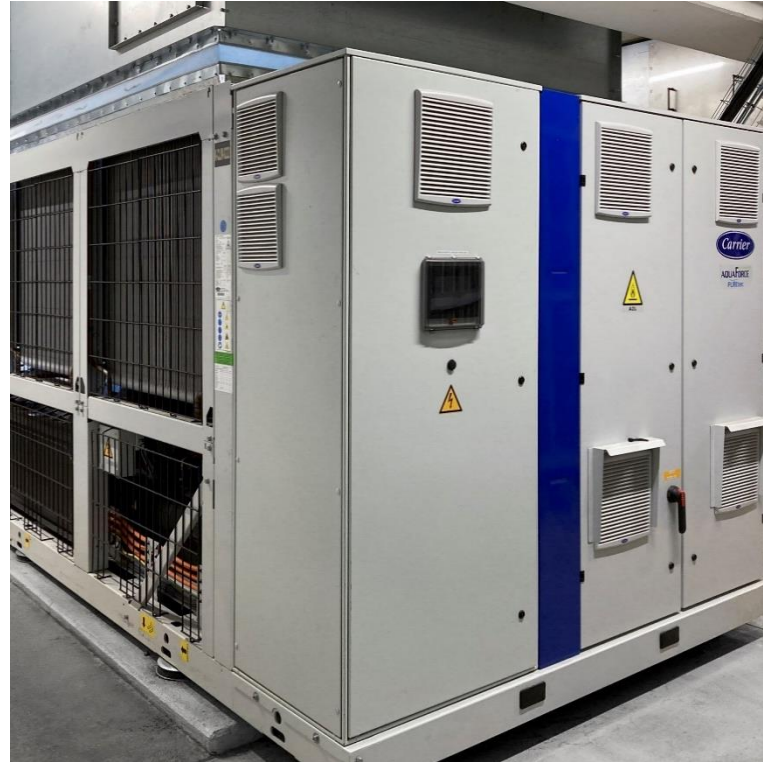
State-of-the-art production equipment Industrial chiller at Kuhn Group, Saverne
