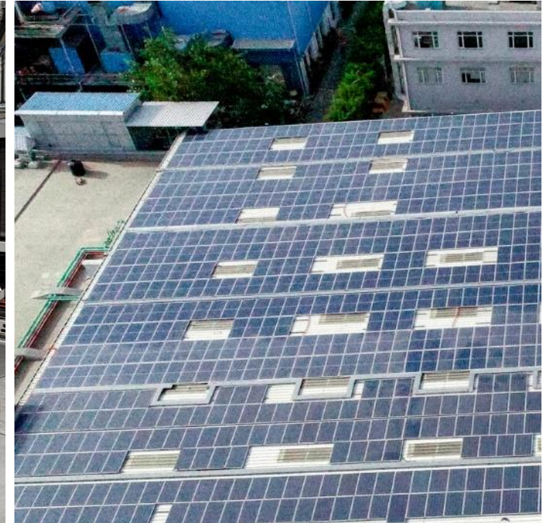
Sustainable power sources Total photovoltaic capacity at kWp 1'224 Solar cells at Bucher Hydraulics, India
