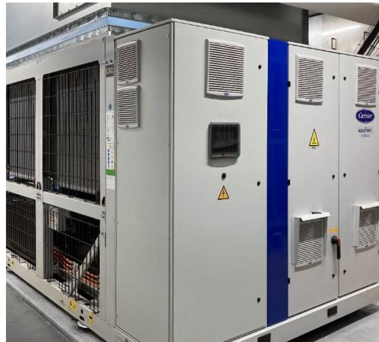
Industrial chiller at Kuhn Group in Saverne
