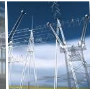
High-voltage switch gear
