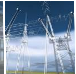
High-voltage switch gear
